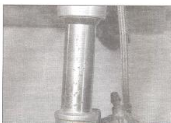
25.5 Corrosion such as this wrecks seals
